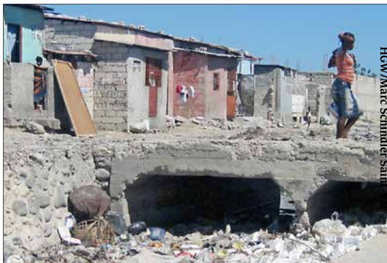
A drainage canal in the Port-au-Prince slum of Cité Soleil. Most canals pass through such poor neighborhoods, emptying human and animal fecal matter, styrofoam, and plastic trash into the Caribbean
