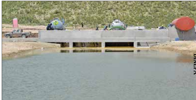
One of the three waste treatment pools at DINEPA's Morne à Cabri site in late 2011, just after it opened. The waste treatment facility is now closed
